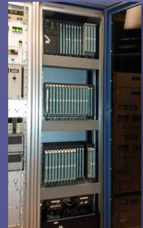
Figure 3. I/O boards in the SCADA system
